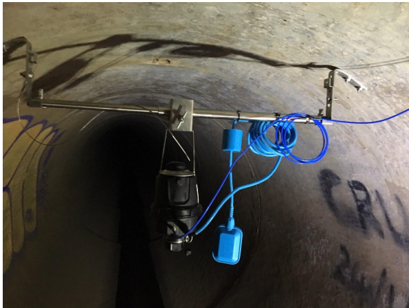
Pollution monitoring equipment installed in stormwater drains
